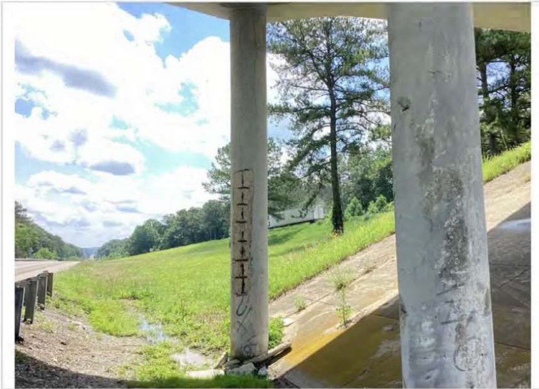
Bent #1 column B spalling
