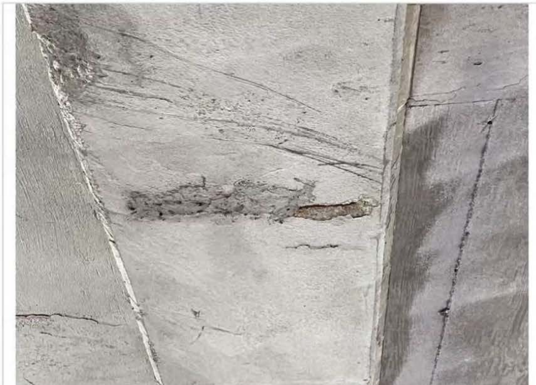
Span 1 beam A spall to steel
