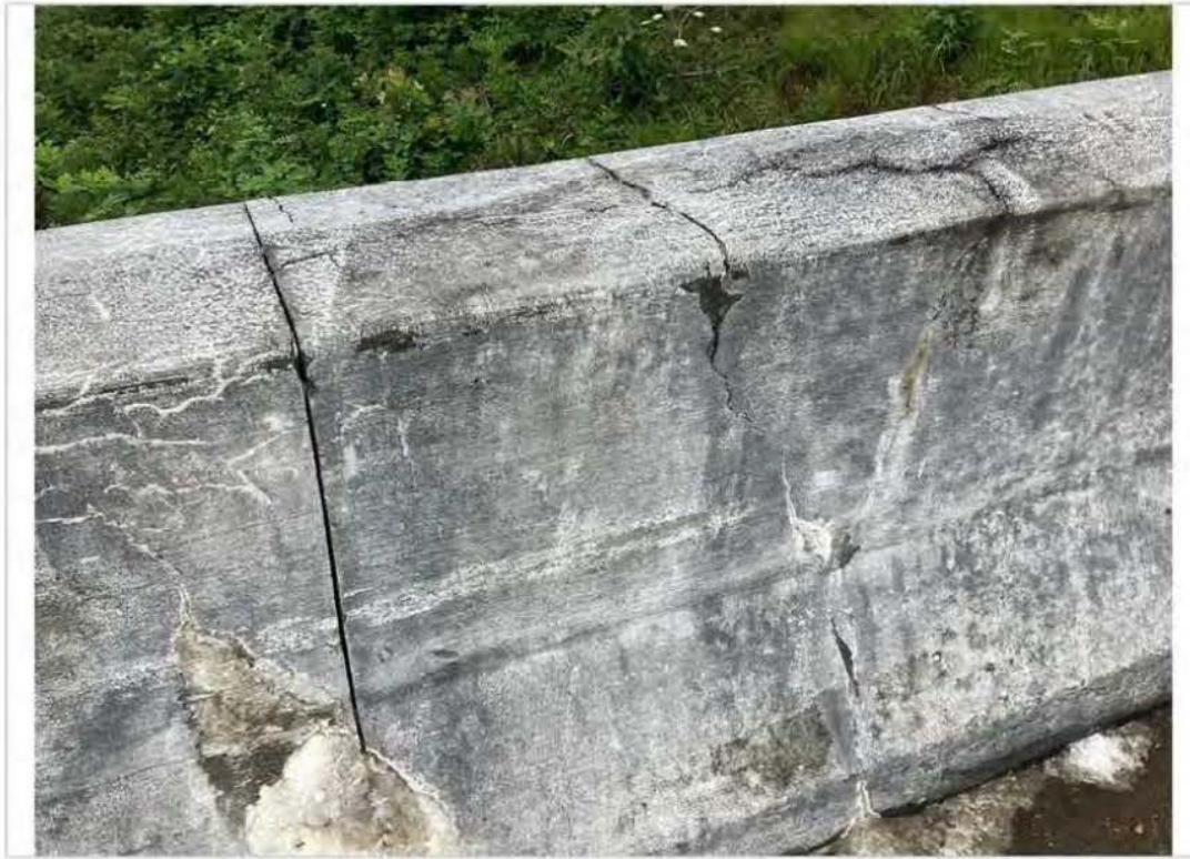
Span 1 parapet crack
