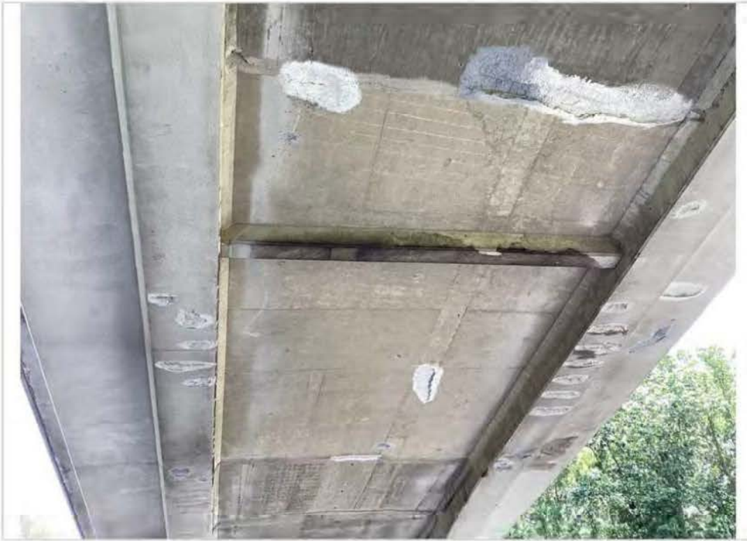
Bottom deck span 2 typical with spall to steel in deck and girders
