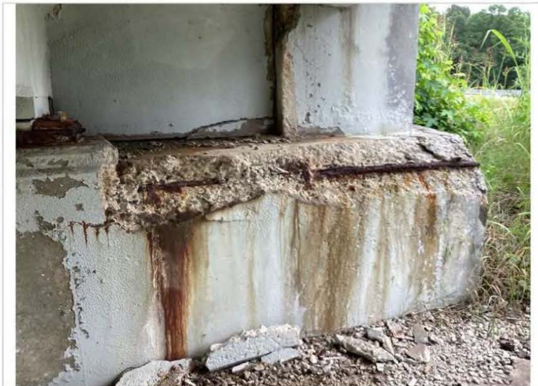
Spall steel abut 2
