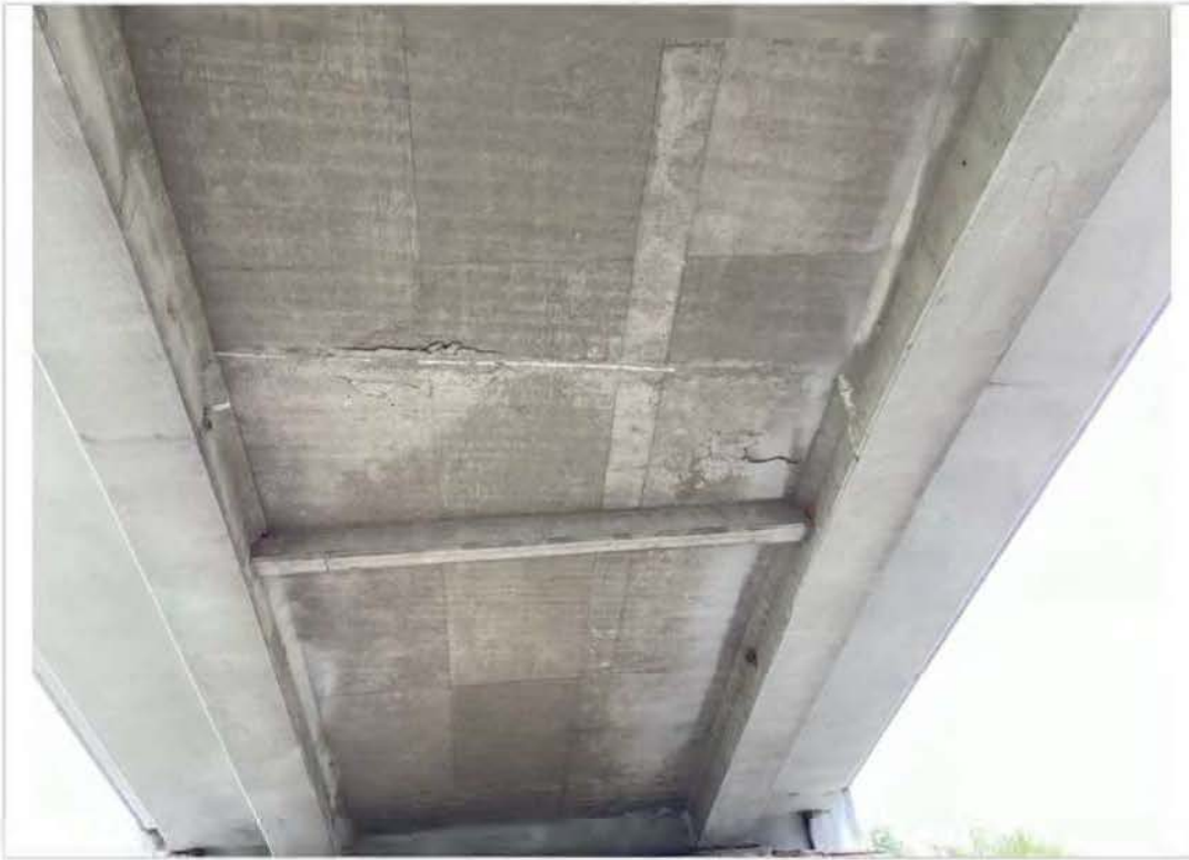
Impending spall on bottom deck of span #3
