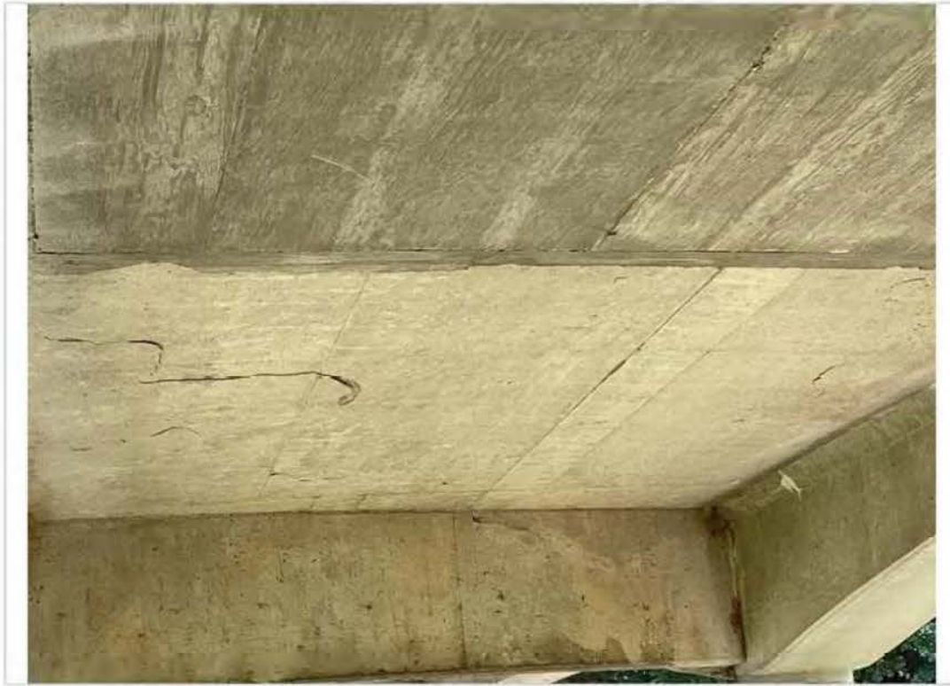
Span 1 bottom deck impending spall typical
