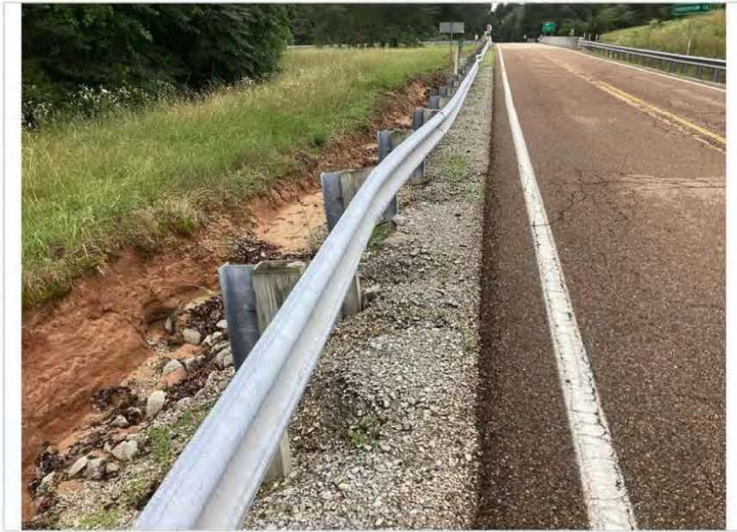
Approach 1 right guardrail damage
