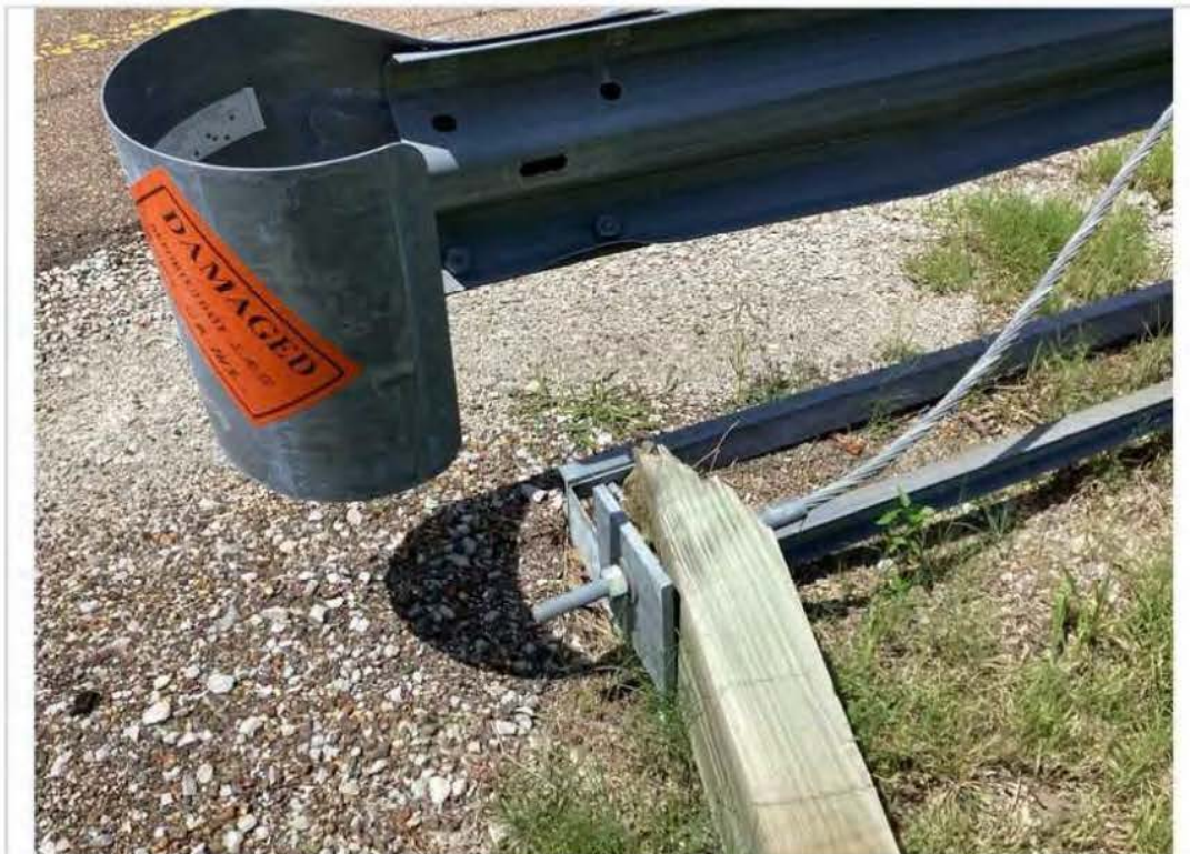
Approach 1 right terminal damage
