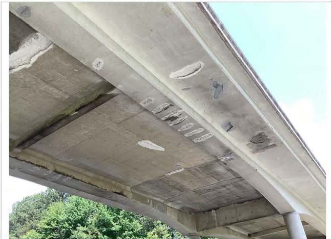
Bottom deck span 2 spall to steel
