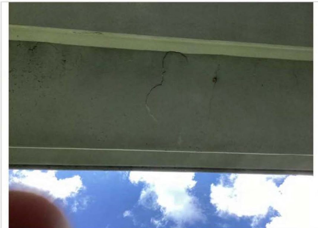
Impending spall on bottom deck of span #3
