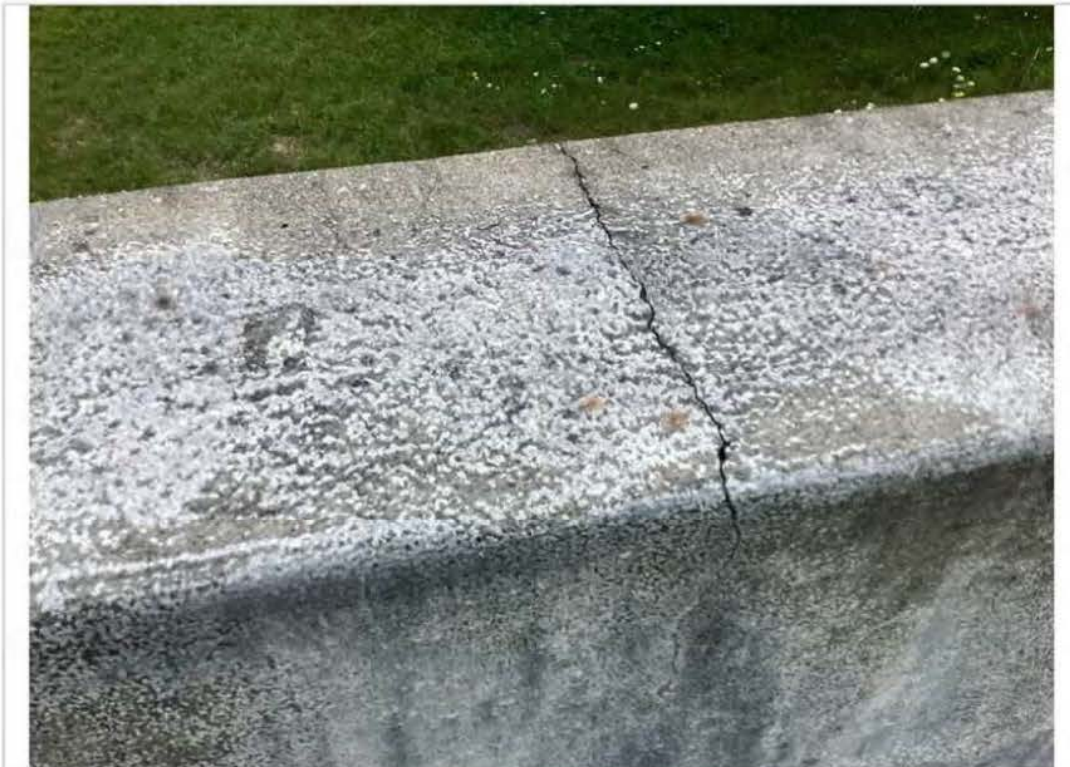
Parapet crack typical
