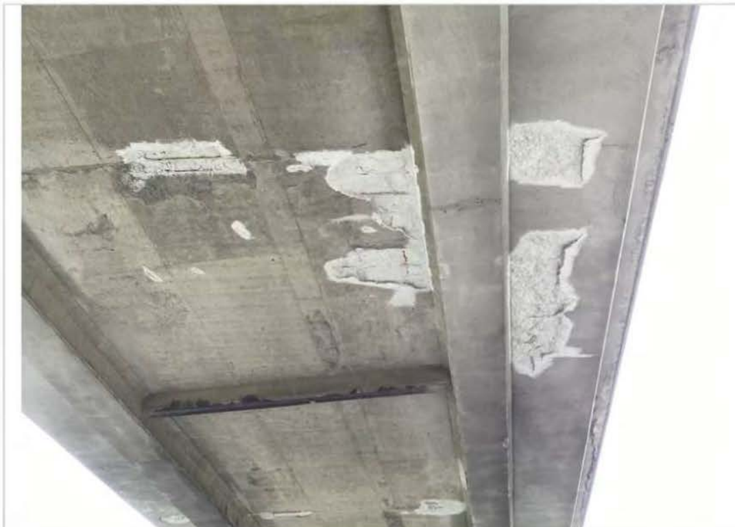
Span 2 bottom deck spall to steel
