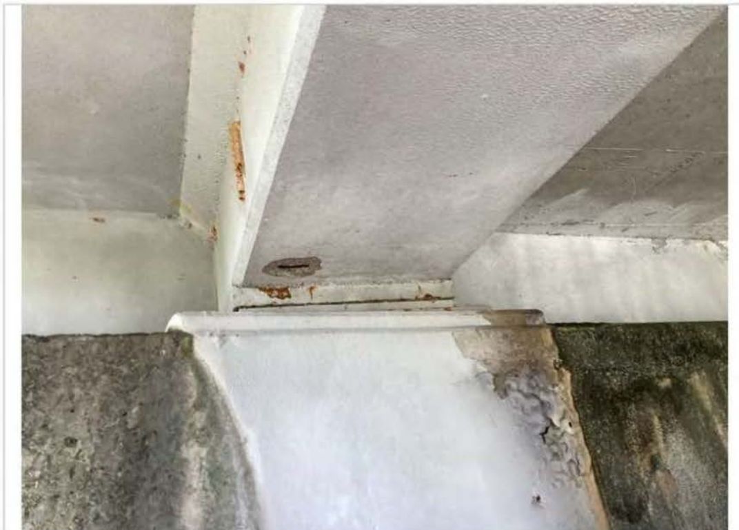
Span 1 beam B spall to steel
