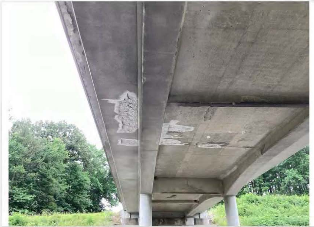
Spall to steel on bottom deck of span #2
