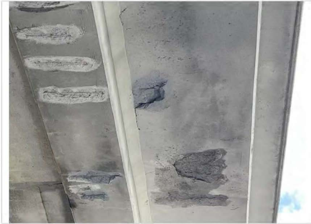
Span 2 right overhang impending spall
