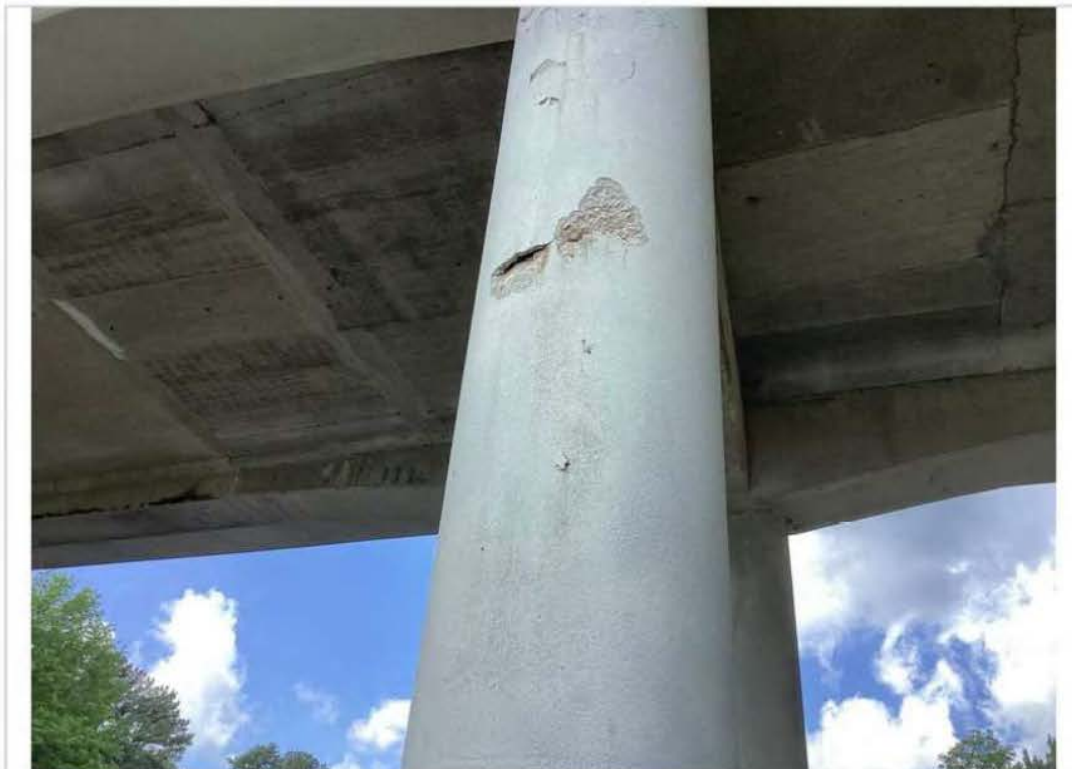
Spall steel bent 1 column b
