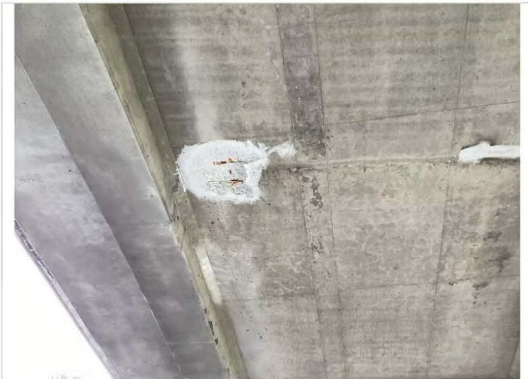
Spall to steel on bottom deck of span #2
