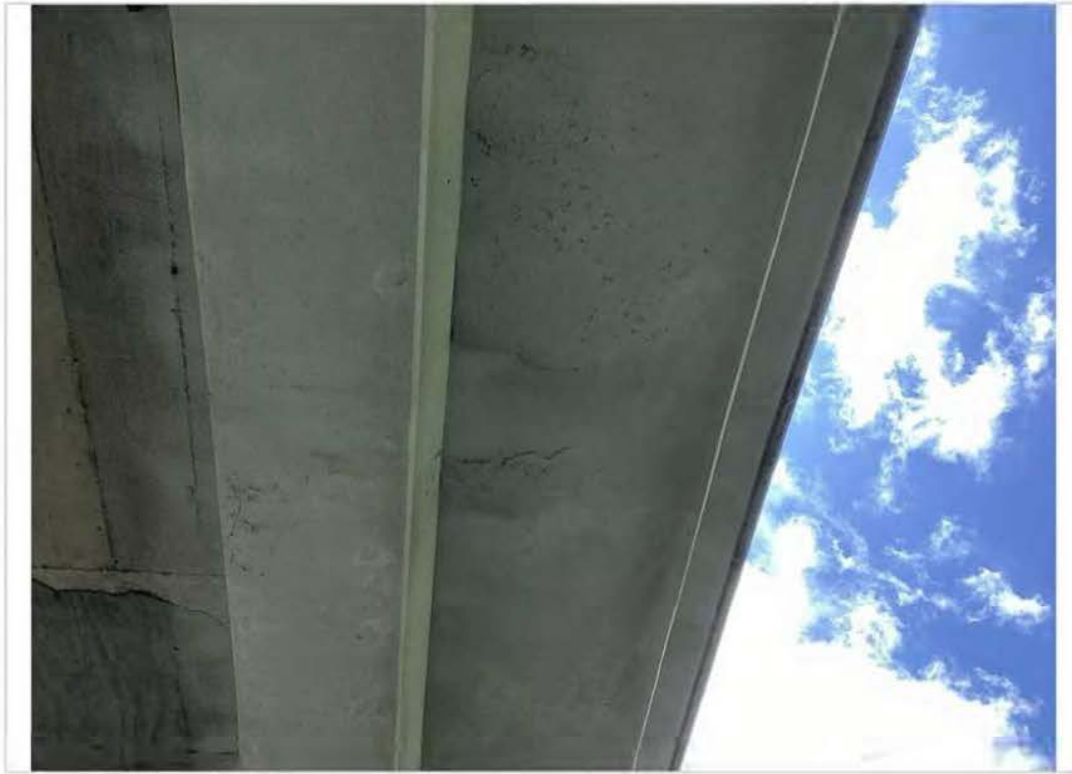
Impending spall on bottom deck of span #3
