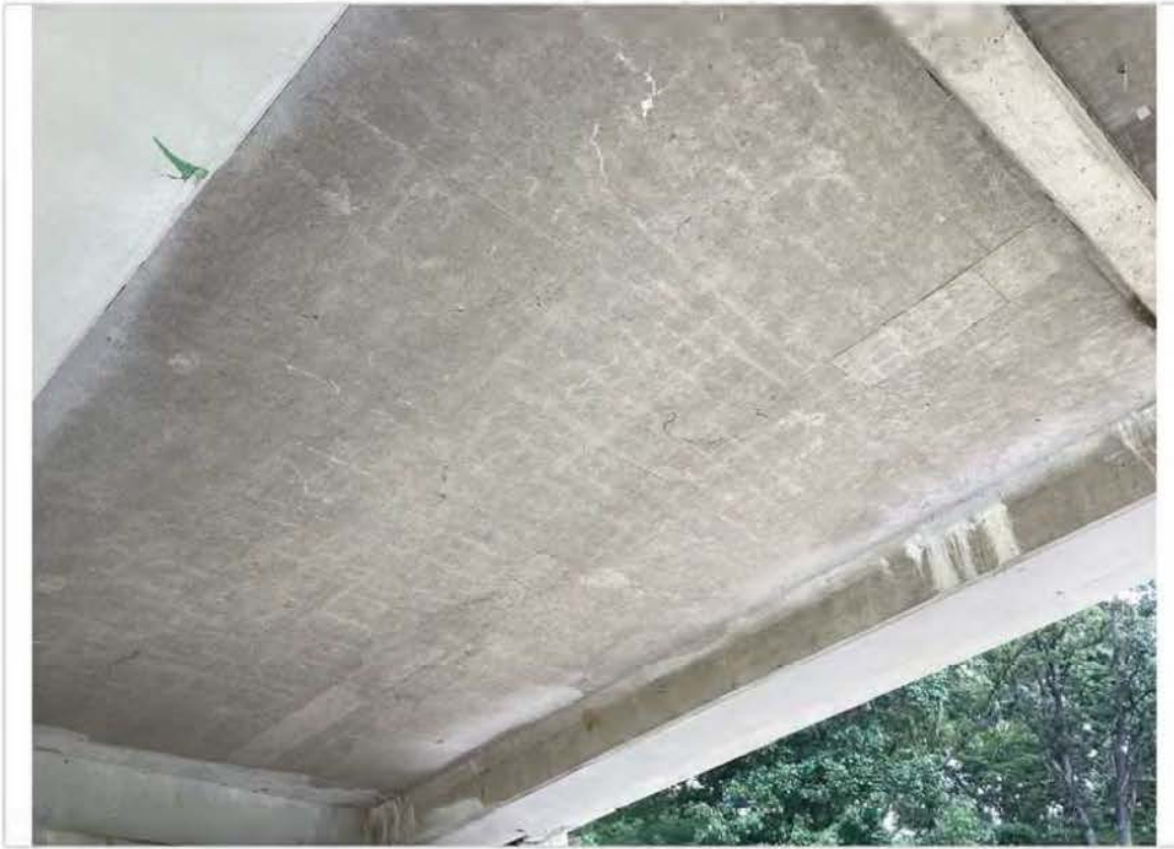
Impending spall on bottom deck of span #3
